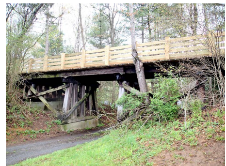
Before/After photos of a now-refurbished trestle on the "first mile" of the Mendota Trail ©Frank Kilgore (1) & Rick Heppert (2)
